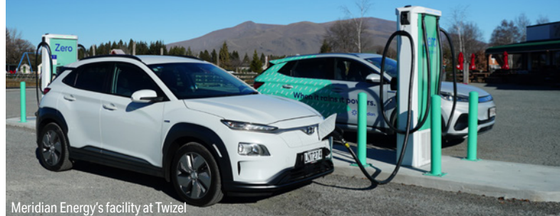
Meridian Energy's facility at Twizel
